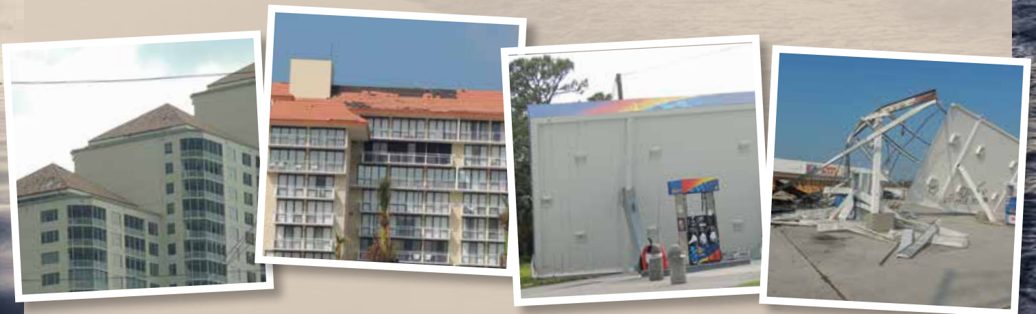
Damage to mid- to high-rise buildings (left to right): Roof tile damage to 20+ story building in Fort Myers, and roof damage to a 10-story building in Marco Island.
