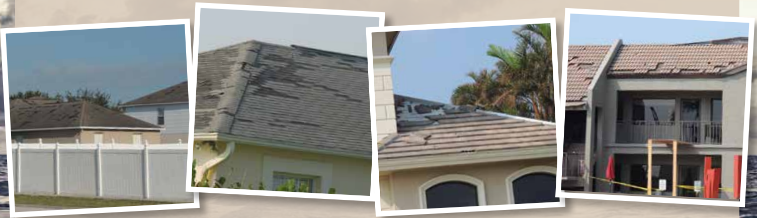
Damage to single-family dwellings (left to right): Roof damage to 2005–2006 built residential single-family dwelling and pre 1998 built home.
